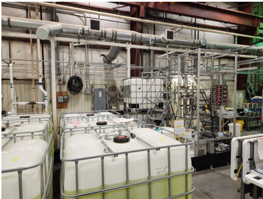
Figure 3.8. Experimental system workspace in PDLE facing west. This is later in the experimental program when the system was in the LS2 configuration and multiple feed simulant shipments had been received (left foreground).
