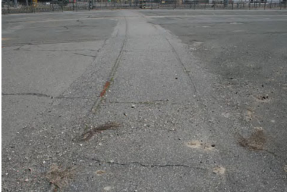
Figure 2-8: Paved Over Rail Spur Originally Connecting the VYNPS Rail Spur Entrance to the Containment Building [6]
