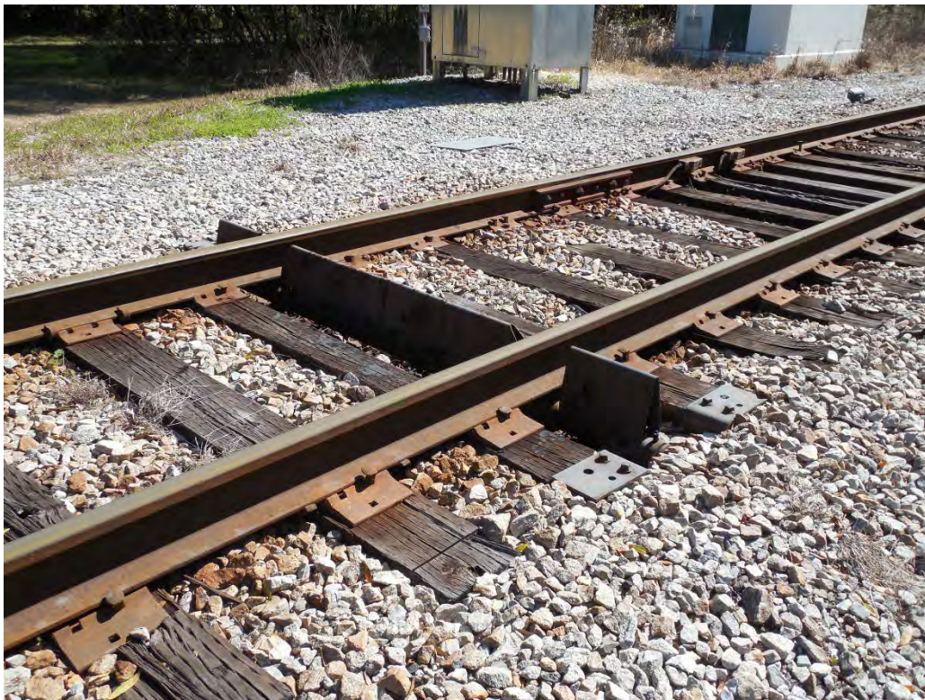
Figure 2-176. Dragging Equipment Detector on Florida Northern Railroad (2015)
