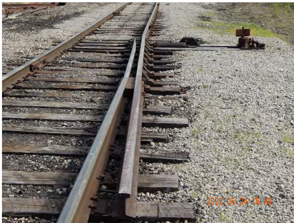
Figure 2-458. Split Derailer on Illinois Subdivision Rail Line
