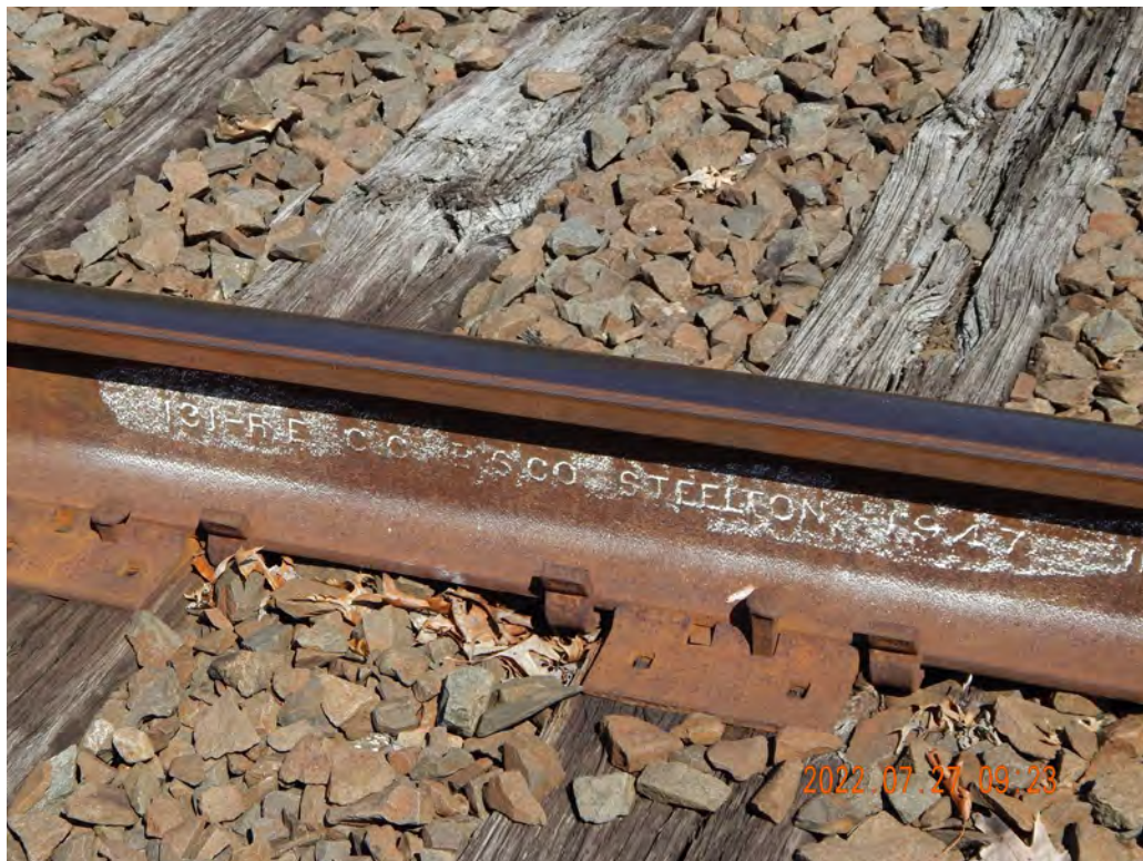
Figure 2-534. 131-lb. Rail Hawleyville Road Potential Transload Location
