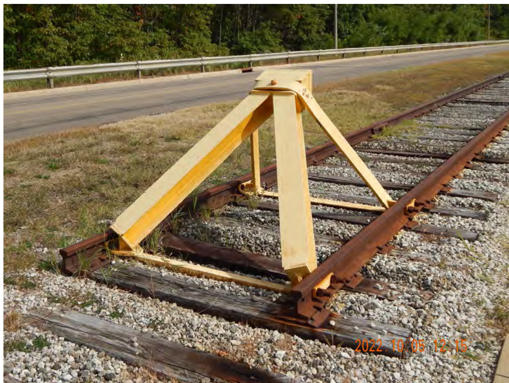
Figure 2-612. Bumping Post on DC Cook Rail Spur
