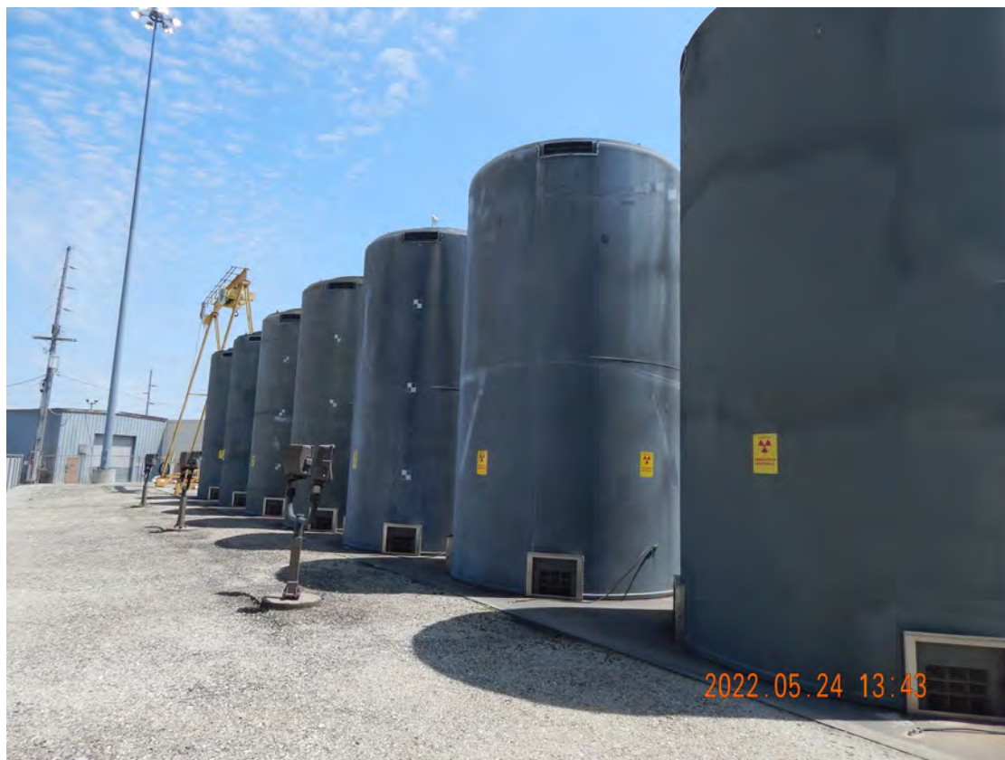
Figure 2-445. HI-STORM Dry Storage Systems at East ISFSI
