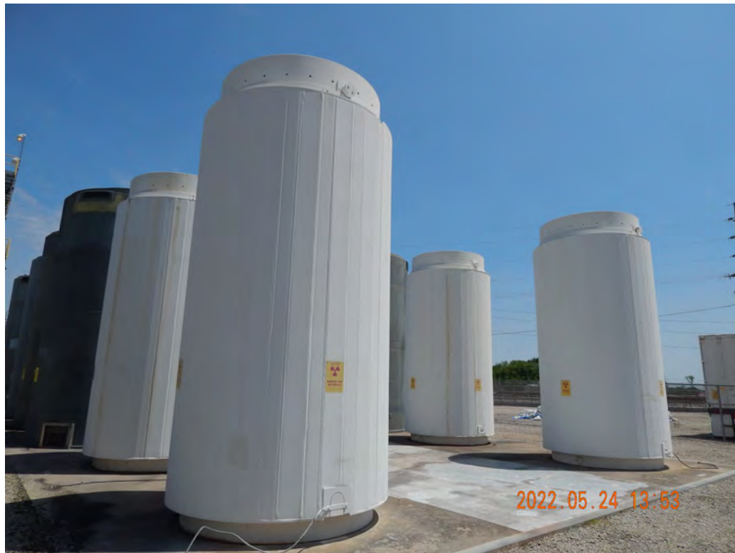
Figure 2-446. HI-STAR 100 Dry Storage Systems at East ISFSI
