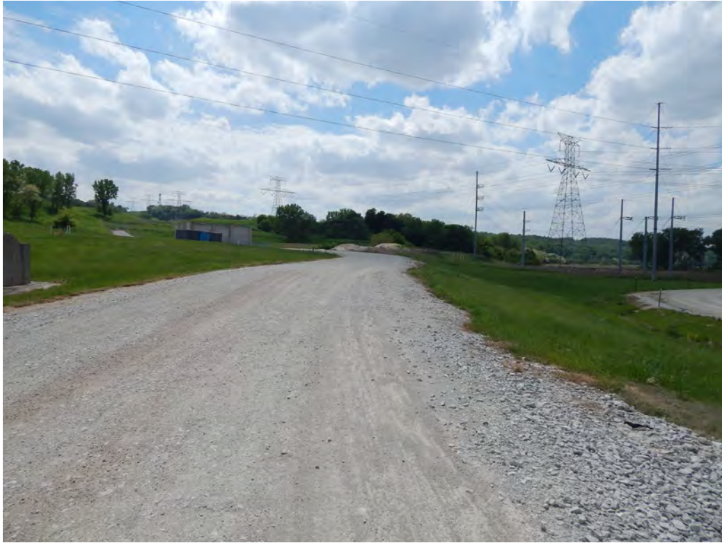
Figure 2-369. Current Condition of Haul Road (2017)
