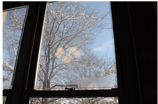
(b) Condensation on the first-floor windows.
