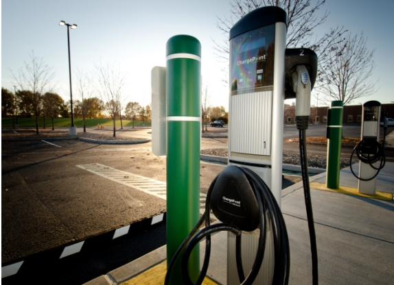
Electric Car Charging Station
